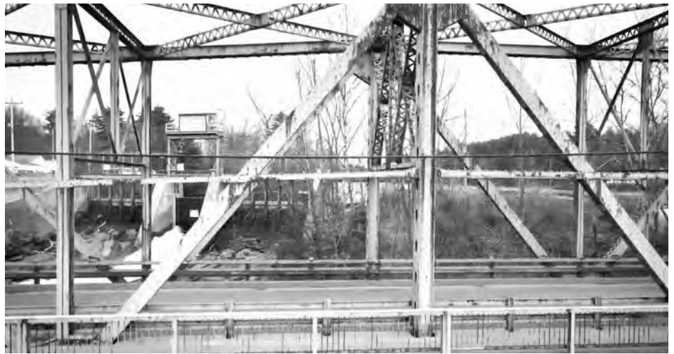
The West Buxton Bridge crosses the Saco River and connects the towns of Buxton and Hollis. The bridge is included in the MaineDOT work plan with construction planned for 2026 and is one of more than 300 structurally deficient bridges in the state.
