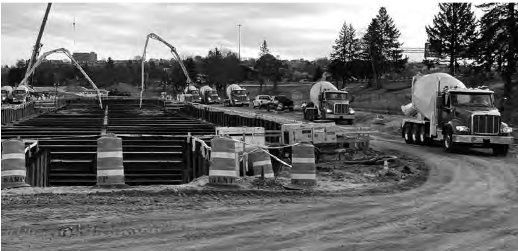
Auburn Concrete trucks deliver concrete to the Portland Back Cove CSO Project for N.S. Gile.
